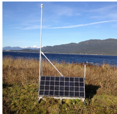
Example of a remote, solar powered AIS site with weather station
